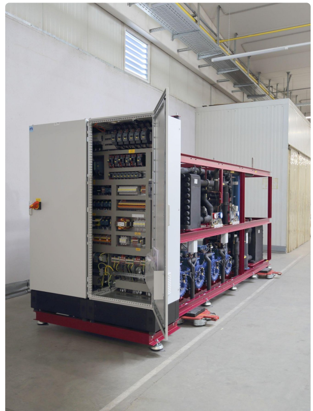
The CO 2 chiller with integrated heat recovery TEKO built for an Italian winemaker. Photo credit: TEKO
